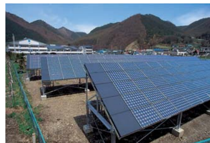
Solar power-generating equipment at Kuzumaki Junior High School
